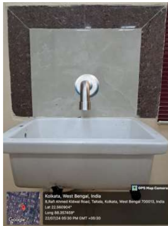
Automatic sensor-controlled faucet within college building
