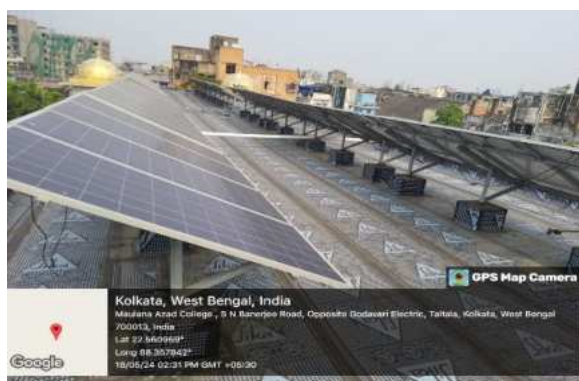
Installed solar panel on college
