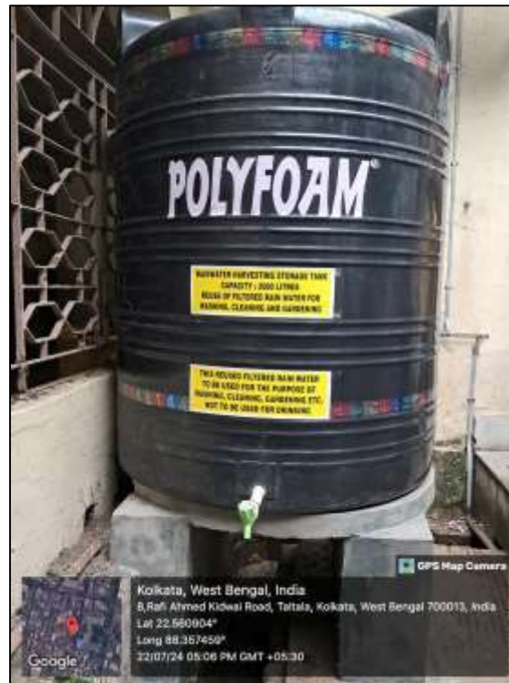
Rainwater harvesting unit 2 for rainwater storage and reuse
