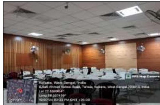
Square LED lights in Seminar hall
