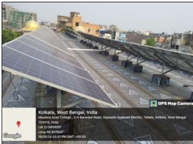
Installed solar panel on college rooftop
