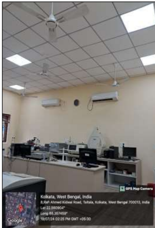
Square LED lights in Laboratory
