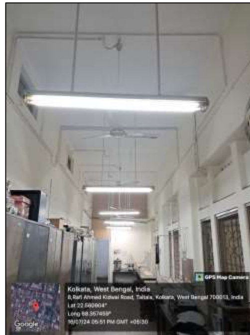
LED tube lights in corridor
