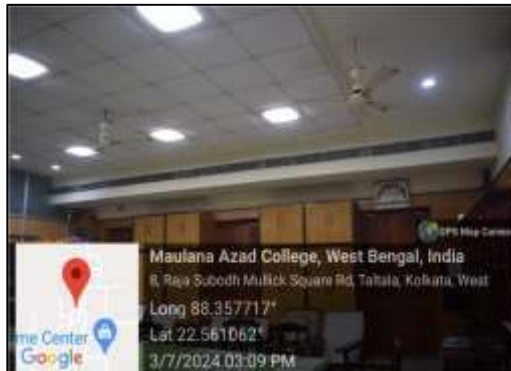
Concealed AC of Common staff room
