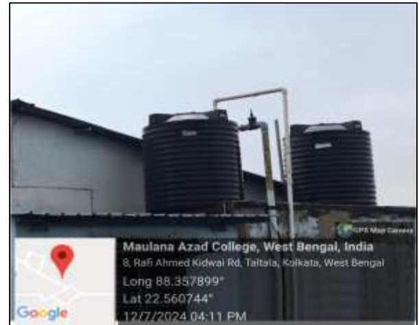
Overhead water tanks in college rooftop
